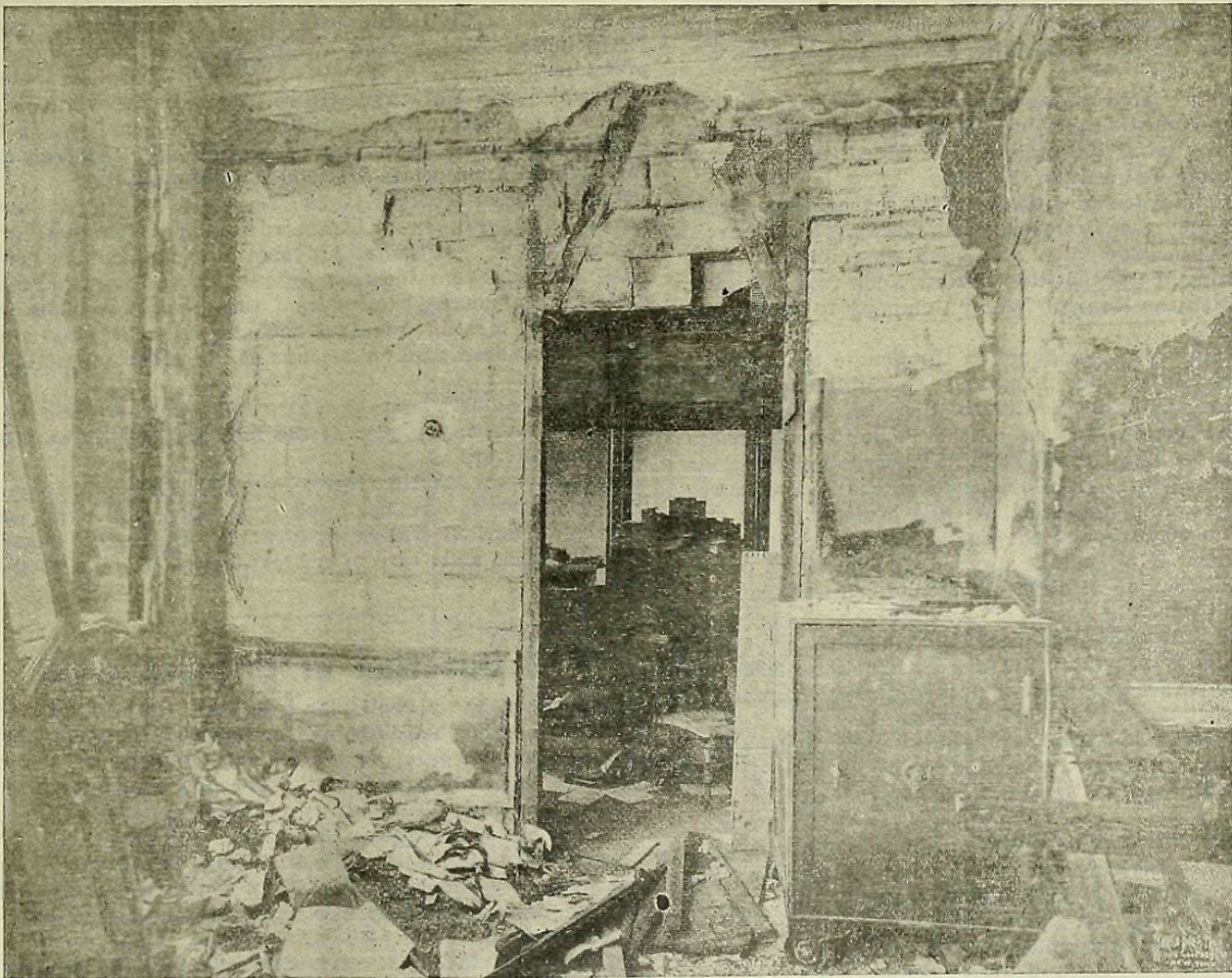
INTERIOR EFFECTS OF FIRE.
